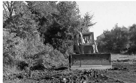
Earth-moving is an integral step in ecological restoration at the Phinizy Swamp Mitigation Bank.
